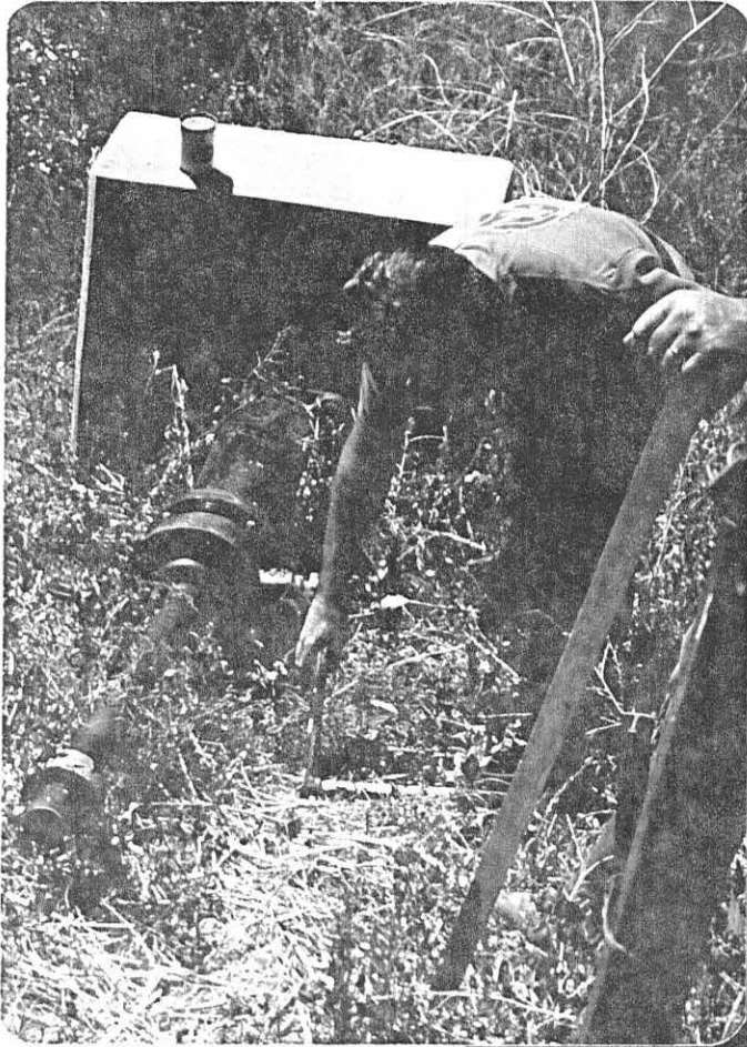
Photo No. 9 Manual operation of the gate screw. Slope of the embankment prevents full turning of the gear with handle.
