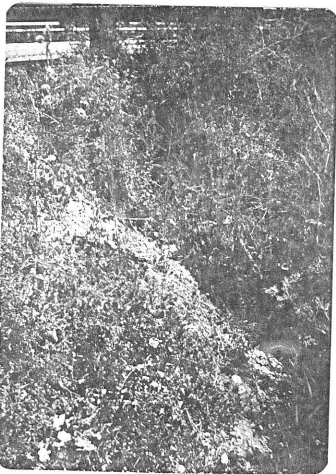
Photo No. 4 Eroded area on upstream slope near crest.
