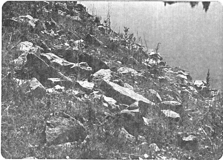
Photo No. 3 Upstream slope, showing misgraded riprap. Typical of entire upstream slope.
