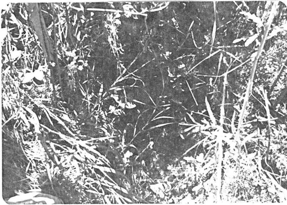
Photo No. 7 Toe drain downstream of left toe, with small amount of water flowing from drain. (Arrow)
