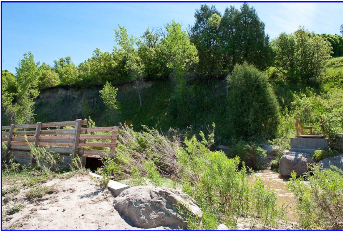
Figure 2: A pedestrian bridge damaged by high flows on Cherry Creek in Castlewood Canyon State Park on the night of June 1, 2009 (Courtesy of Tim Tonge).
