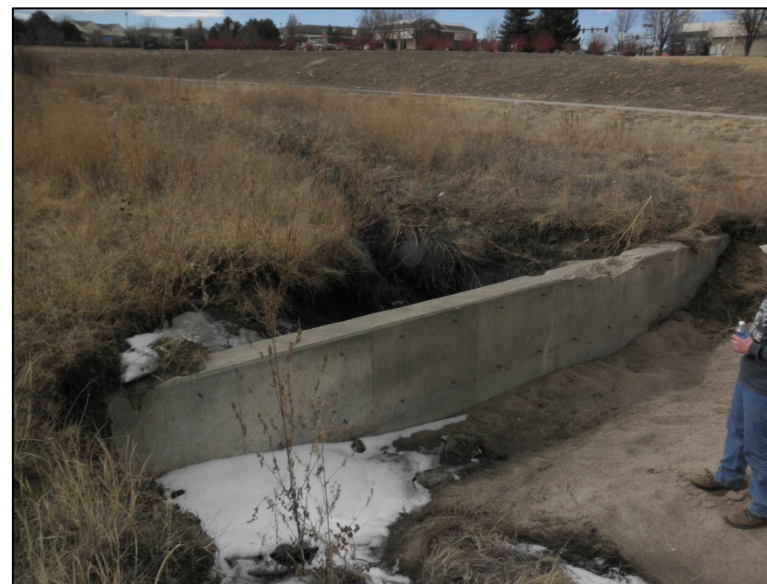
Degradation and Scour at Existing Check Structure
