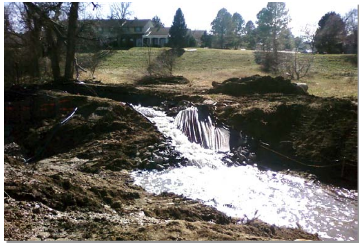
Photograph TDC-1. Use of a temporary diversion channel (right side) to enable installation of a grade control structure (left side). Photo courtesy of WWE.
