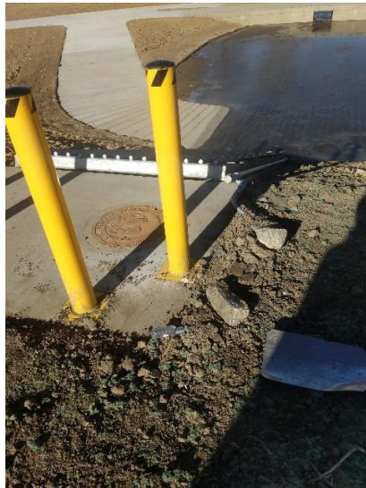
Figure 3: PT well point for Niver Detention.
