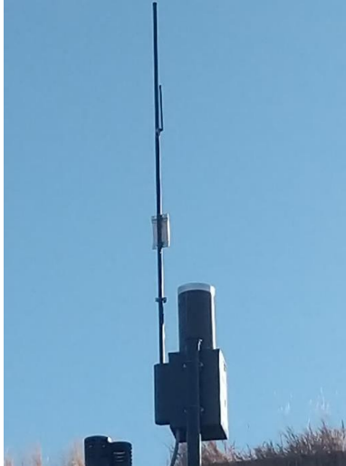
Figure 2: Niver Detention cabinet enclosure.
